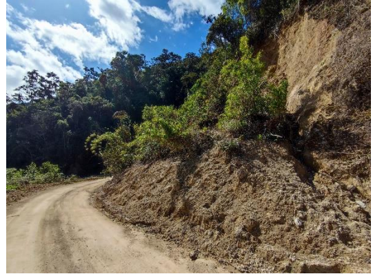
Talud natural inestable
