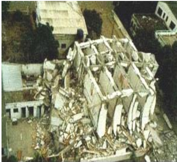
Total collapse of a 6 story RC building
